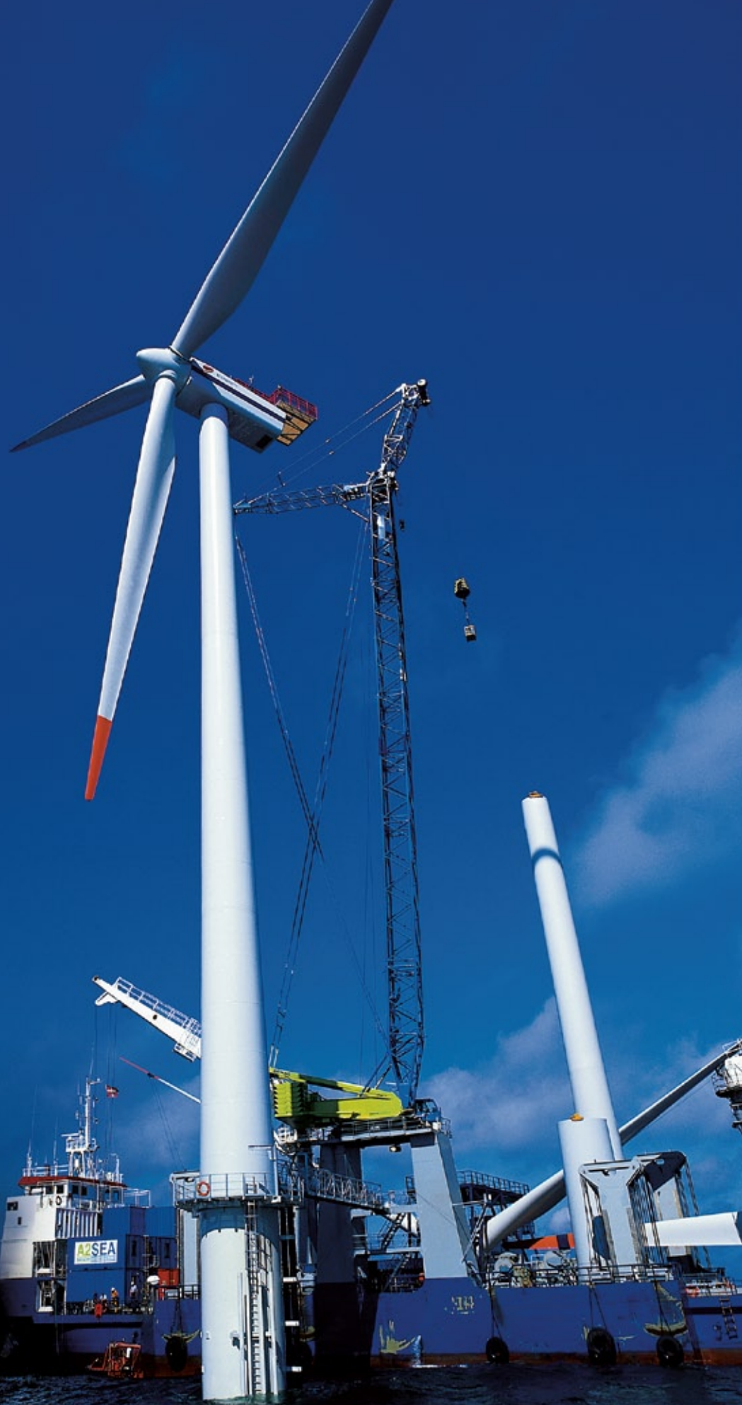
Construction of the Horns Rev I offshore wind power plant in Denmark
