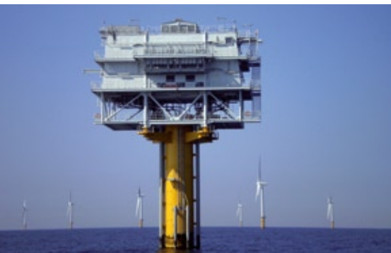
High voltage station for the Prinses Amalia offshore wind farm / Netherlands
