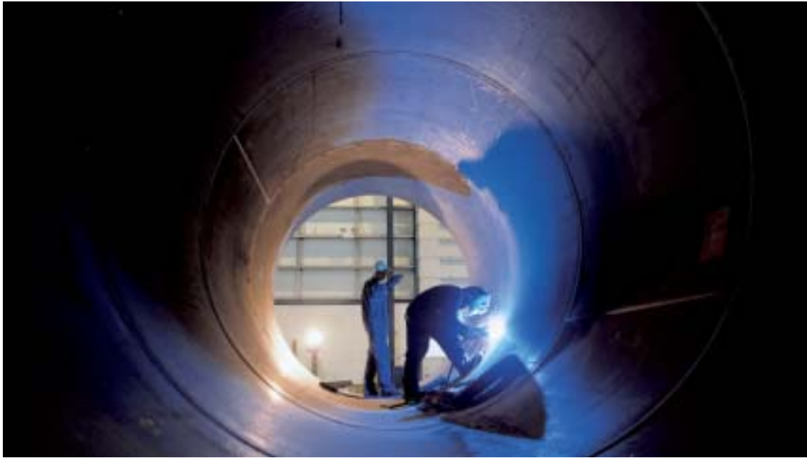
An energy management project was implemented at the tower factory in Varde, Denmark. The project has provided Vestas with valuable experience as regards energy-saving initiatives.
