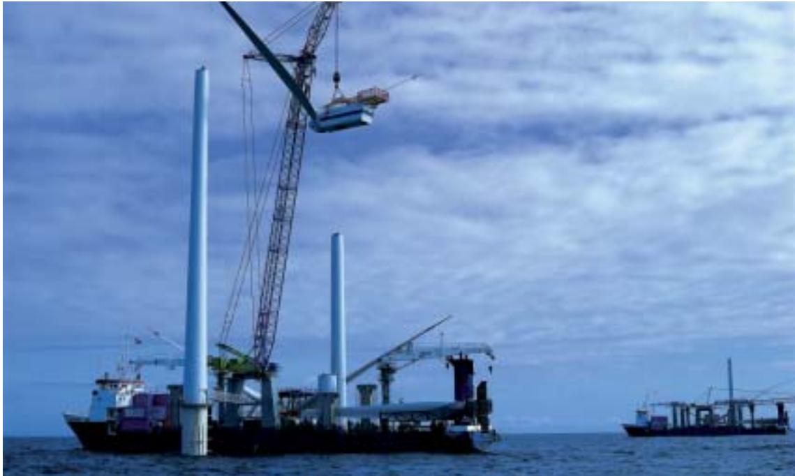
In order to erect the offshore turbines at Horns Reef as quickly as possible, Vestas utilised a technique that required only four lifts to complete the installation.
